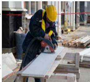
Protected worker cutting fiber-cement board using a circular saw with dust controls
