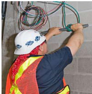
Using hand tools or spare bits of pipe eases stress to the hands while pulling wire.
