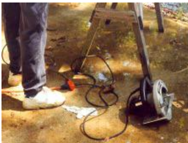
Combinations of hazards increase risk.
