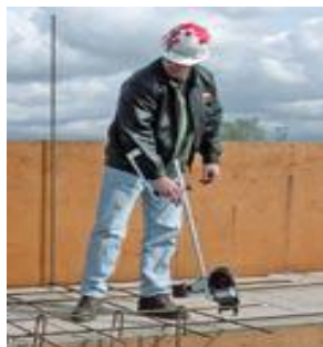
Use a rebar tying machine. It allows workers to tie while standing upright.
